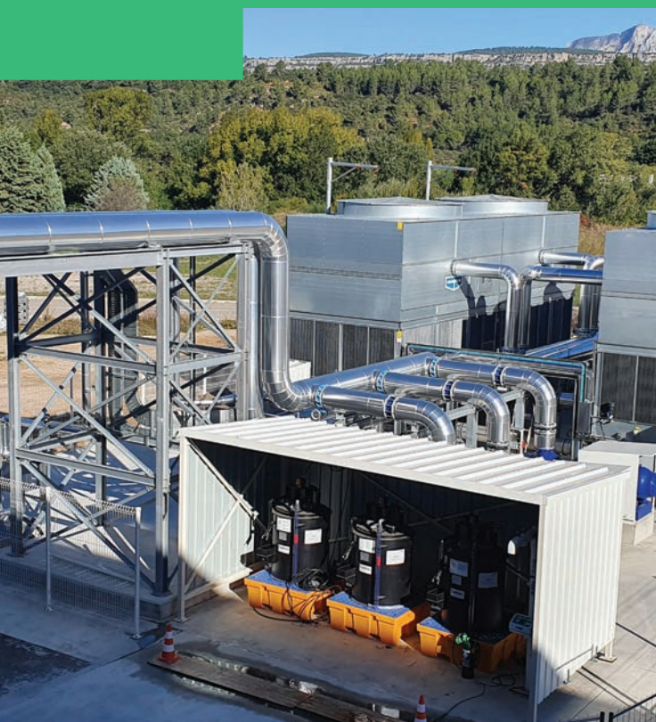
Installation de refroidissement "aero free cooling", ST Rousset (France)
