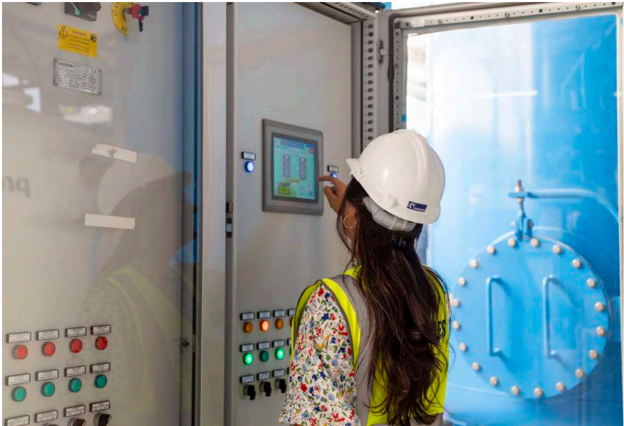
Control Panel of the Reverse Osmosis System
