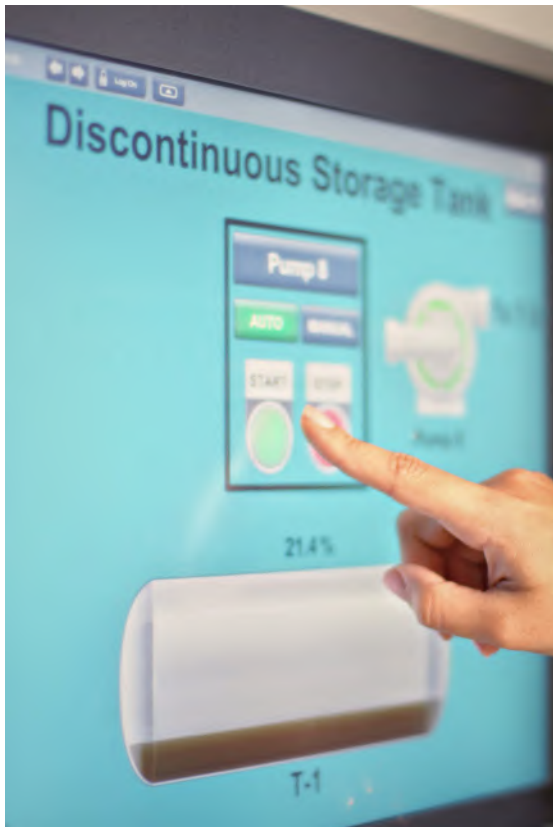
Detail of the WWTP Controller
