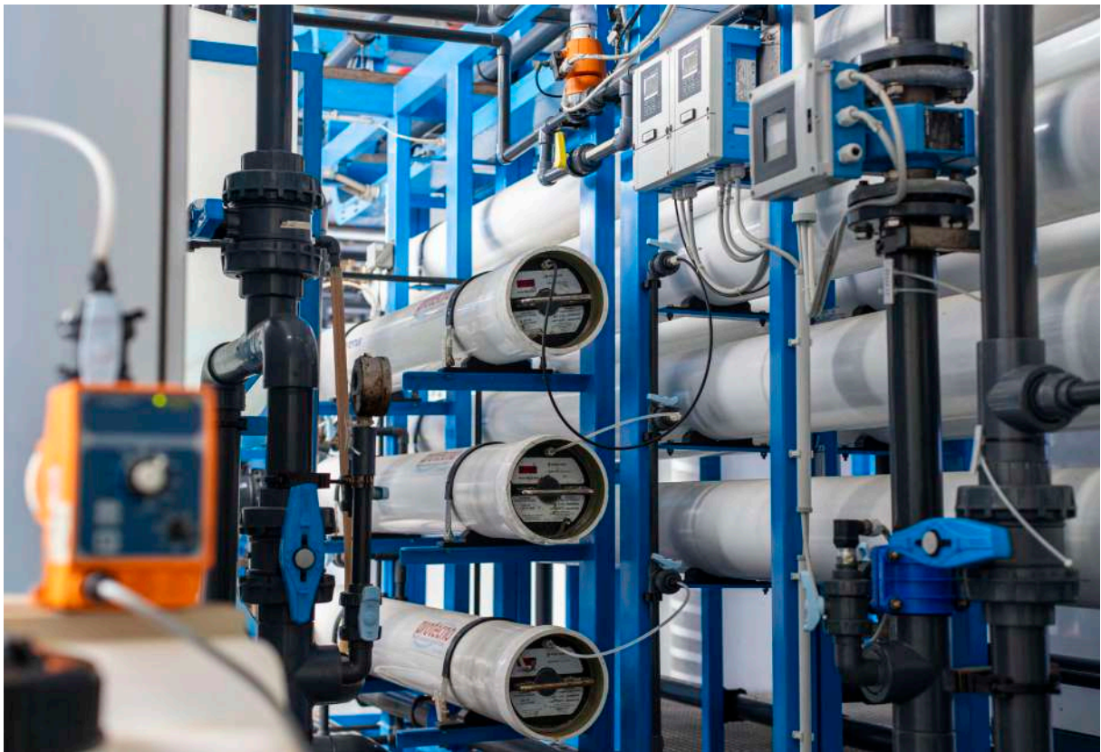
Reverse Osmosis Water Plant
