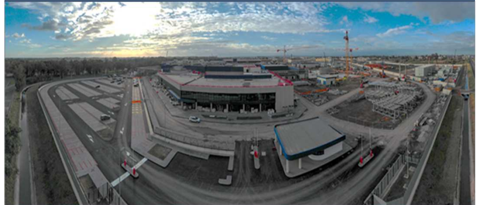
Catania new integrated SiC plant
